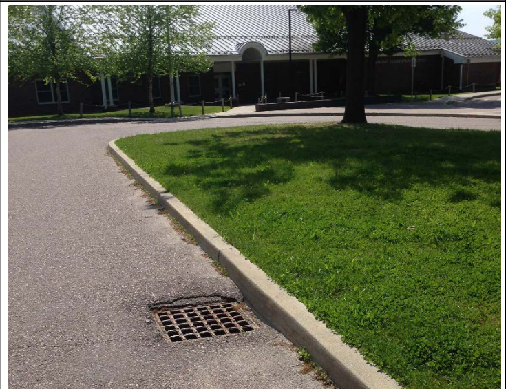
Photo 2. Potential overflow location at existing catch basin.
