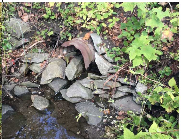
Photo 2. Corroded and undersized culvert
