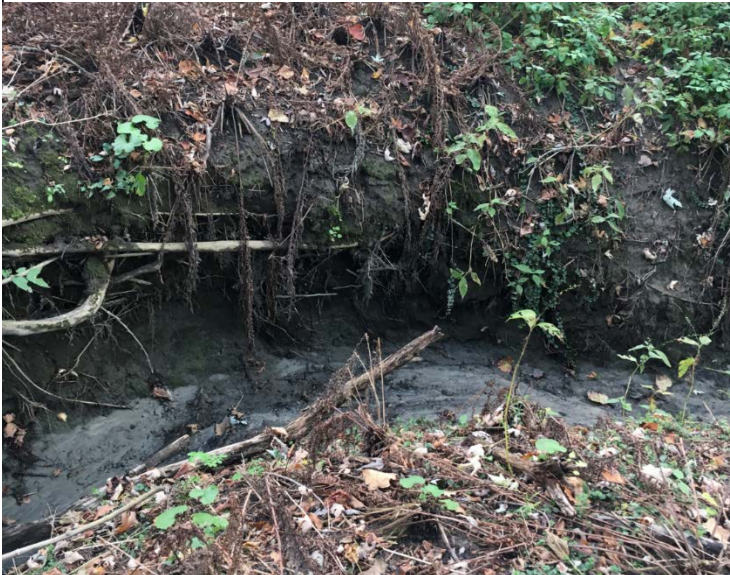
Photo 1. Eroding drainage ditch
