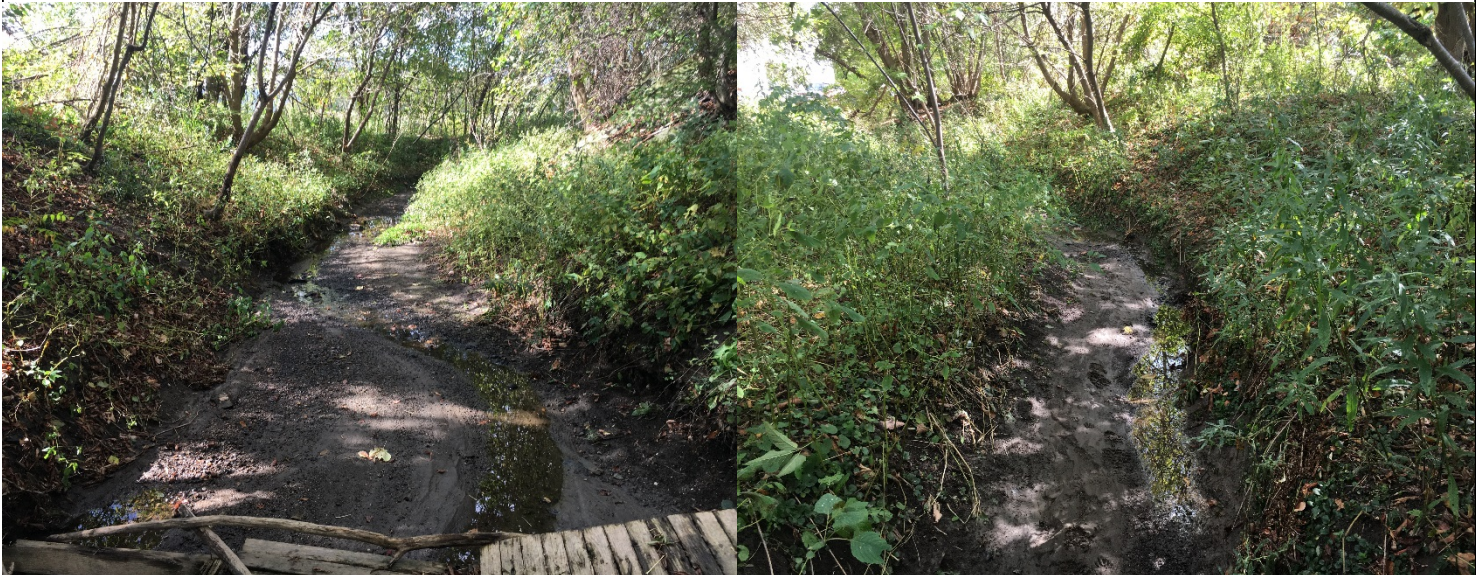
Photo 1. Eroding drainage ditch down-slope of existing outfalls.
