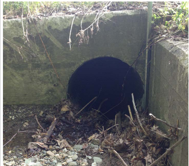
Photo 2. Culvert inlet intercepting intermittent stream flow and upland runoff from the F2 drainage and conveying it beneath I-89.
