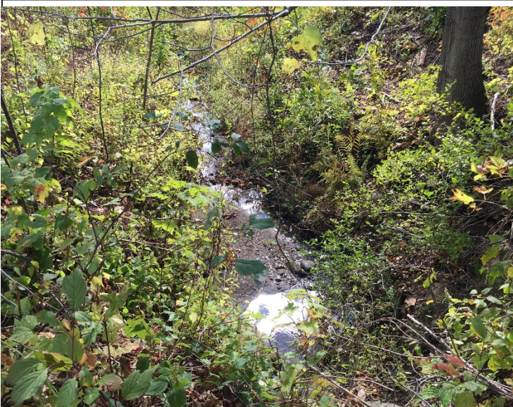
Photo 1. Eroding drainage ditch and sediment transport
