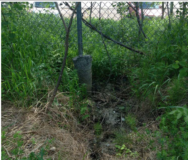
Photo 1. Gully erosion downslope of culvert outlet, leaving I-89 ROW and entering USD 17 property. Note exposed concrete fence footer and chloride-damaged vegetation.
