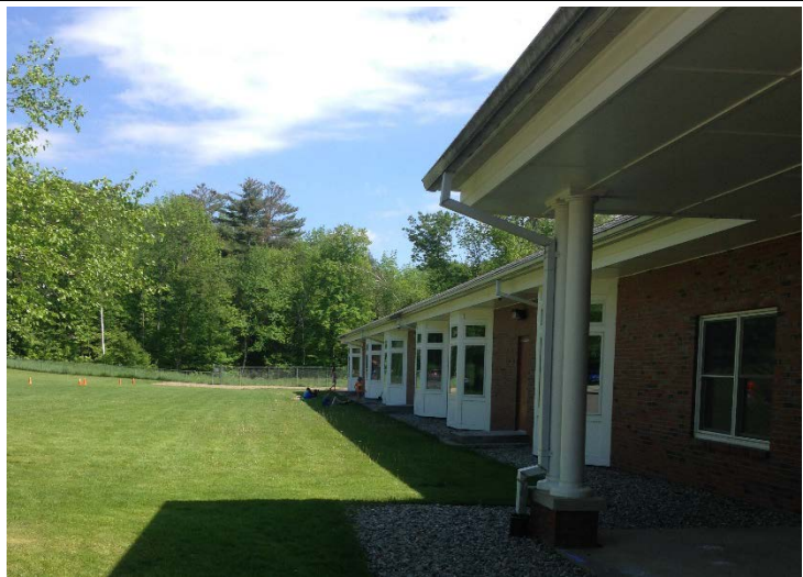
Photo 1. Proposed rooftop disconnection area, also showing existing gutter and drain system for roof fumoff.
