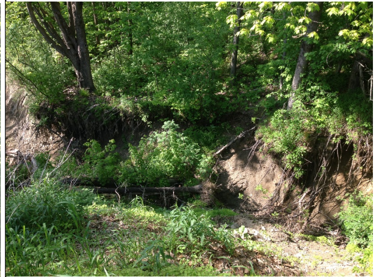
Photo 2. Same gully wall as Photo 1, showing recent erosion and a large tree toppled into the gully with leaves still green.
