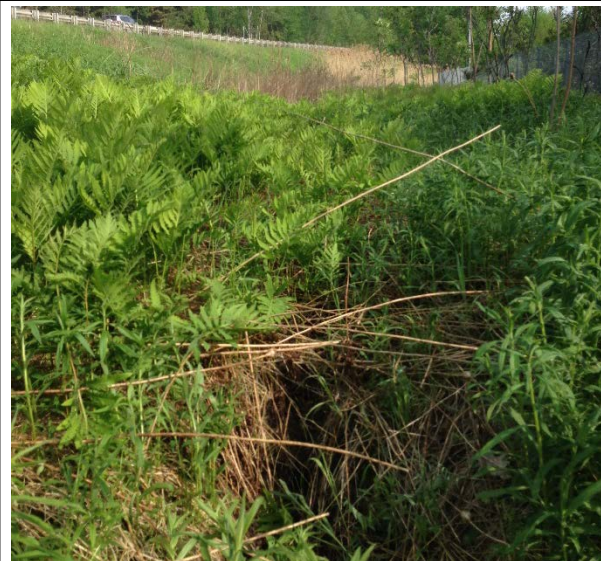
Photo 2. Potential treatment area within the VTrans ROW downslope of culvert outlet. Note erosion in the foreground, which joins gully erosion from culvert outlet and reaches USD 17 property.
